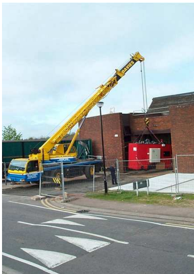
Compte 700kW boiler installation in progress, image courtesy of Worcestershire County Council
